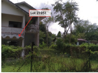
View 2 - Current Site Condition of Lot 21951, Kg Mata-mata Showing of Existing Abandoned House to be demolished facing from front side from Simpang 52-19, Jln Mata-mata
