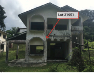
View 1 - Current Site Condition of Lot 21951, Kg Mata-mata Showing of Existing Abandoned House to be demolished facing from front side from Simpang 52-19, Jln Mata-mata
